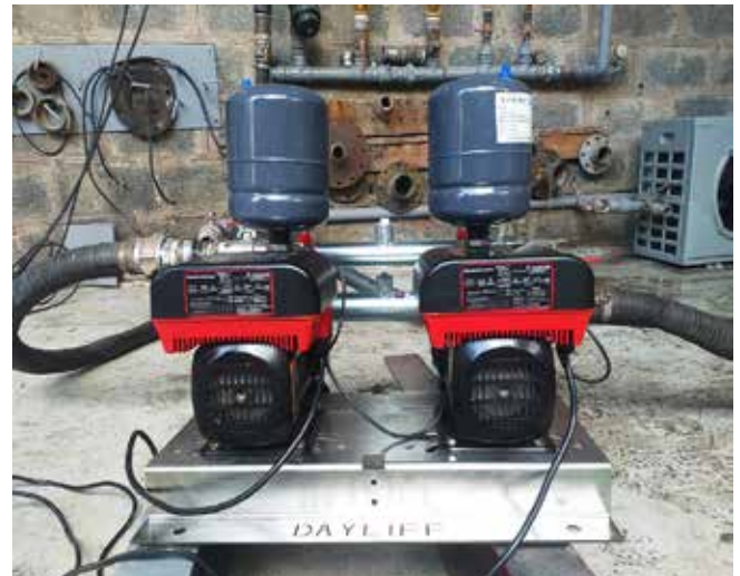
Twin Pump setup under workshop testing
