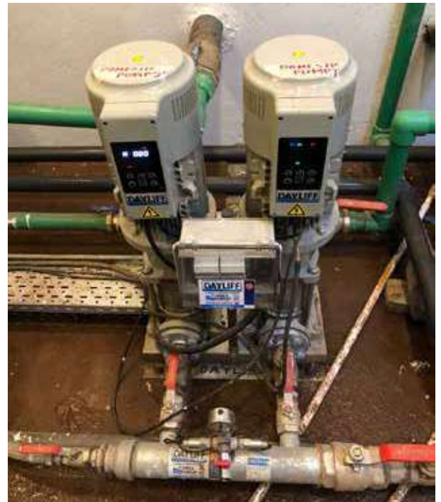
DIX smart pumps installed at a 43 unit apartment block on General Mathenge Drive
