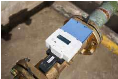
Boiler Hot-water Meter
