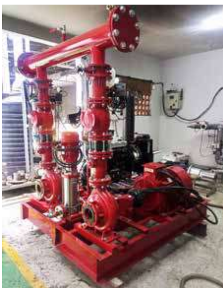
Fire Set undergoing workshop testing
