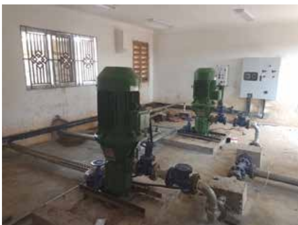
Rovatti Multistage Pumps Installed in the pump room at Kifura
